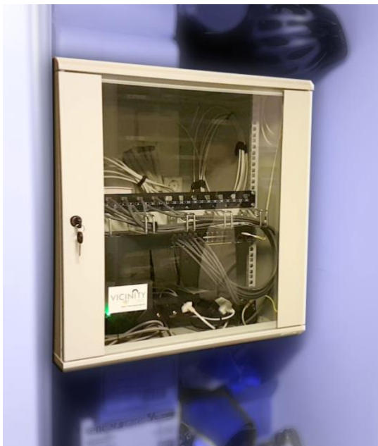
Figure 10: Locked steel closet for equipment
