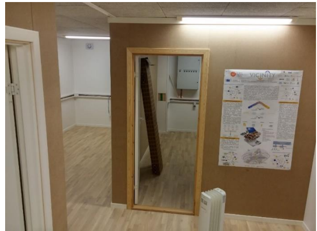
Distribution AC and DC rings installed around the IoT house
