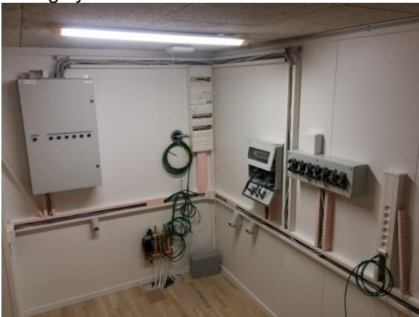
The Electrical DC & AC installed Panels
