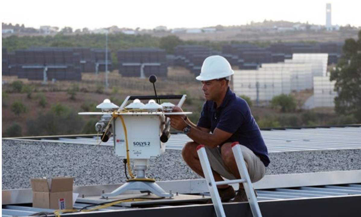
Installation of UV-E sensor at SOLAR Lab 1
