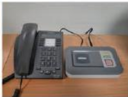
Data Center Communication
